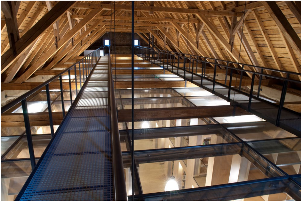
View of the Main Hall from the Castle Roof Truss © Ing. arch. Jaromír Kročák
